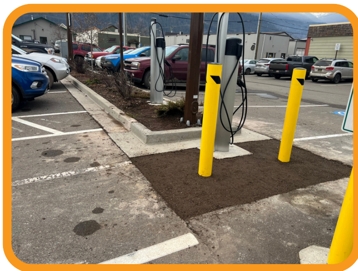
EV Charging Stations
