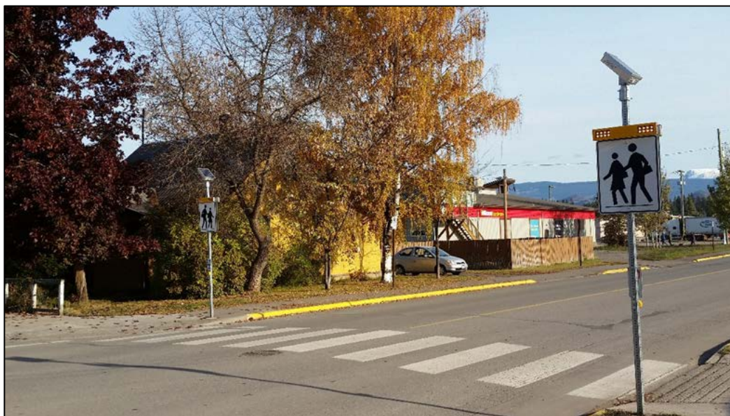
Solar-powered LED Flashing Beacon Crosswalk Signs on King Street at Second Avenue
