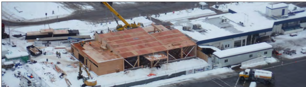
Photo (below): Expansion of the Smithers Regional Airport Expansion Project in progress.
