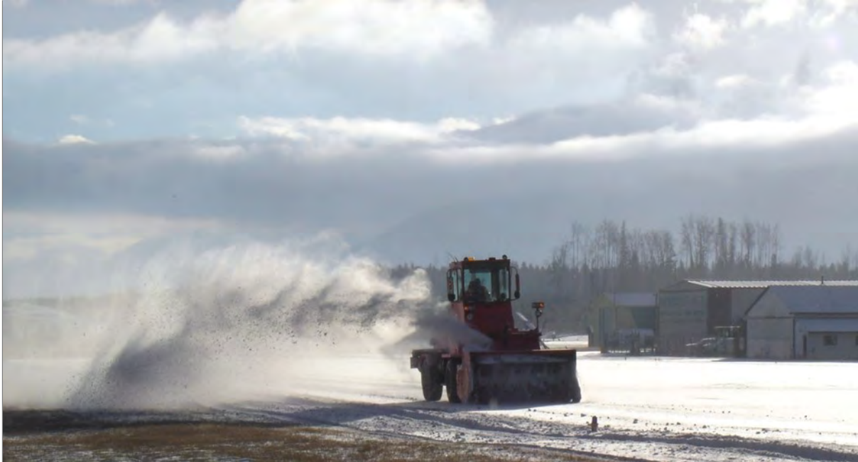
Photo Above: The Sicard snow blower sprays snow 100 feet from the edge of the Airport's apron to allow aircraft to safely manoeuvre to load/unload passengers and freight.
