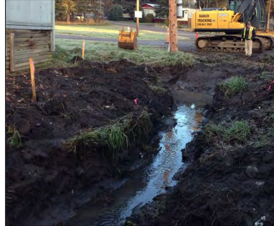
Photo Above: Astlais Place - Hudson Bay Mobile Home Park Drainage Channel Cleaning
