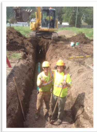
Photo: Members of the Works and Operations Crew working on a storm sewer connection in a residential area
