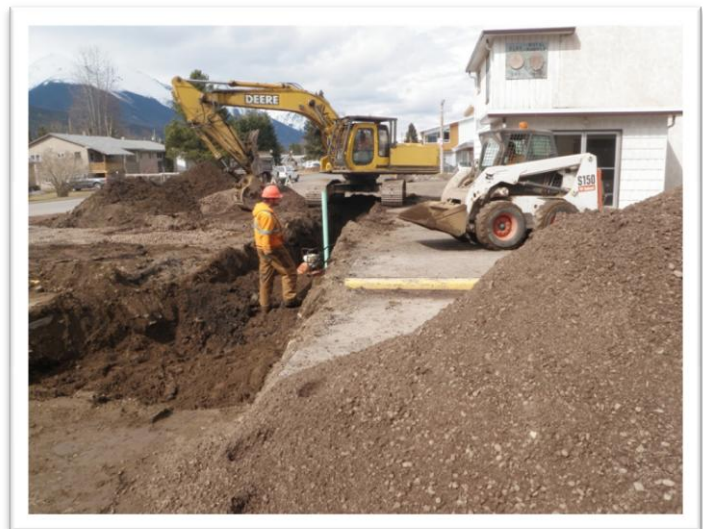
Photo: Works and Operations Crew working on a storm sewer connection in a business area
