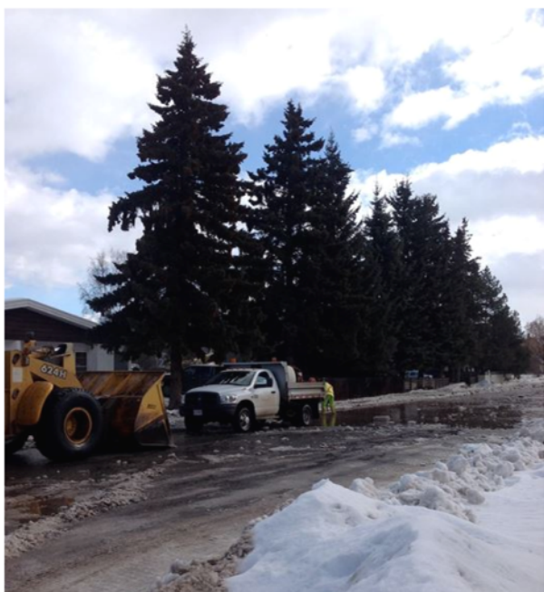
Spring Ice Removal from Catch Basins
